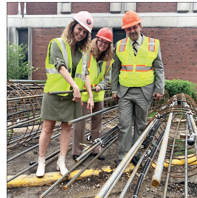
Dr. Tugce Baser, Morgan White, and Dr. Mohamed Attalla at the site of geothermal piles in the foundations of the CEE bridge
